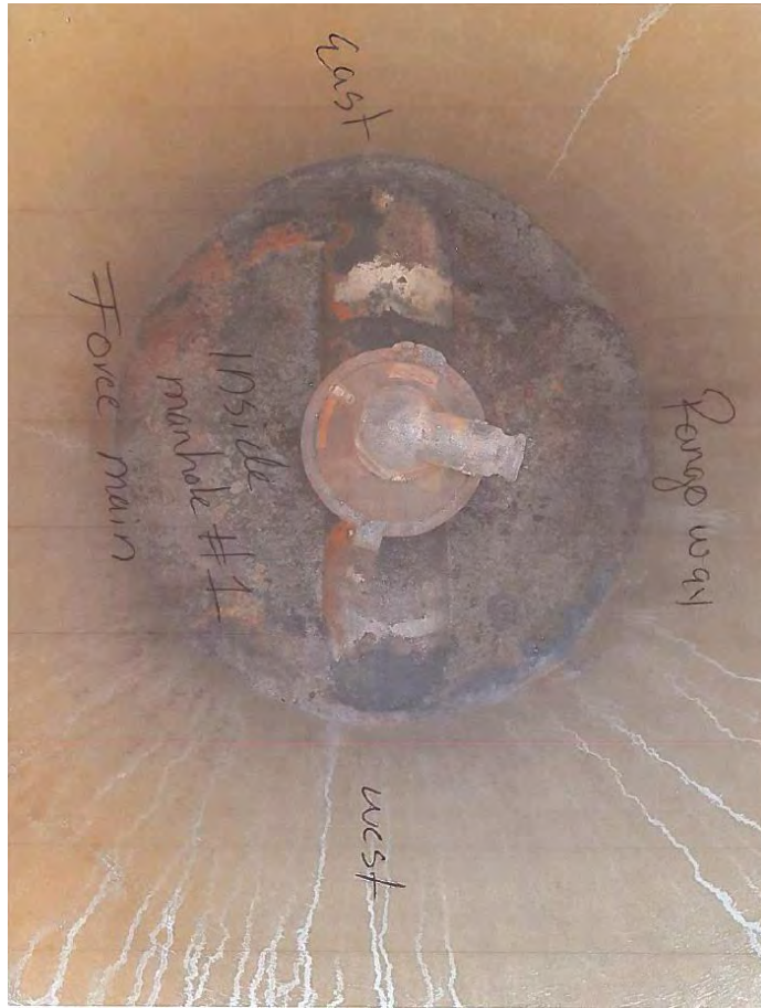
Figure 4-2: Air Relief Valve in Manhole 1F
