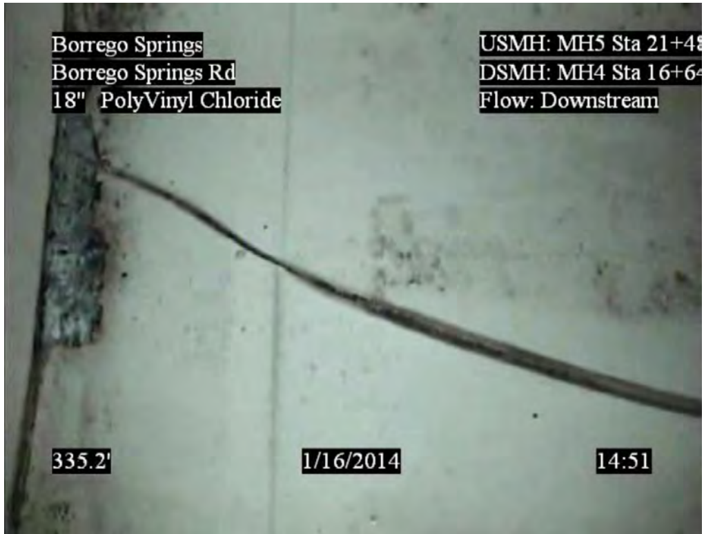
Figure 5-4: Longitudinal Crack in Gravity Main Segment E (1 of 2)
