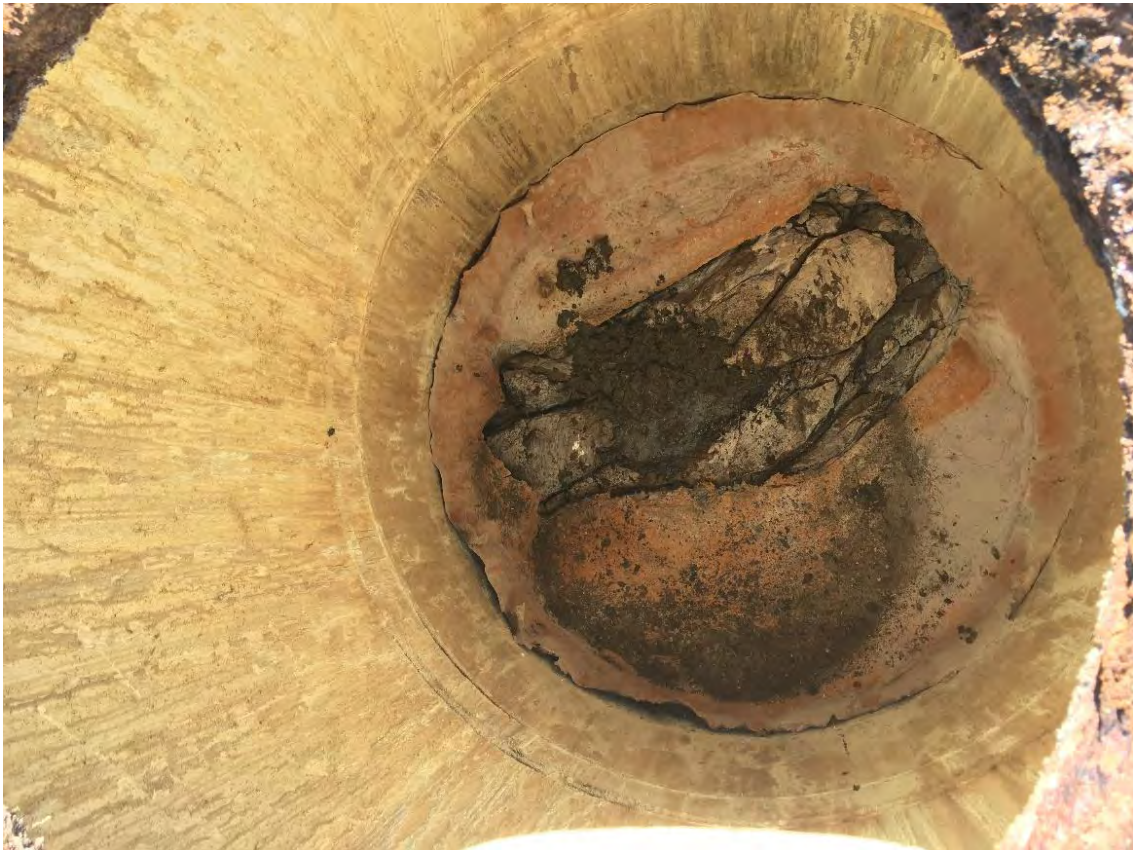
Figure 5-3: Solid Deposits in Manhole #9
