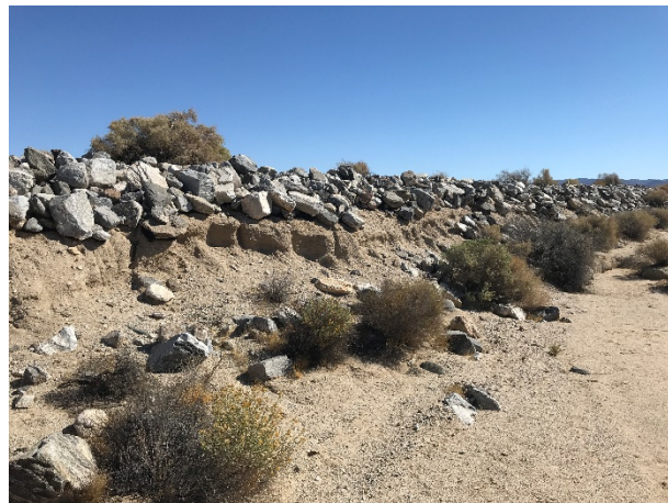
Photograph 8 – Berm erosion causing displacement of riprap (Site 8).
