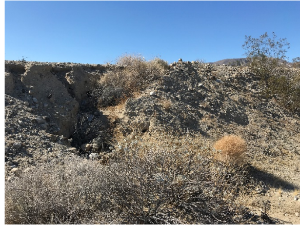
Photograph 2 – Gully erosion of earthen berm (Site 2).
