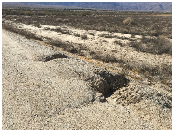
Photograph 14 – Gully erosion in earthen berm (Site 16).
