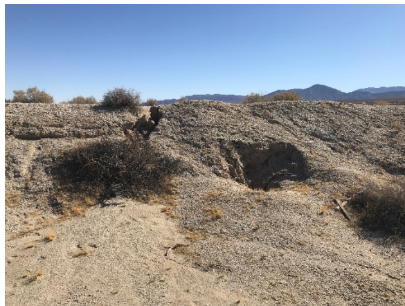
Photograph 12 – Hole and gully erosion in earthen berm (Site 12).
