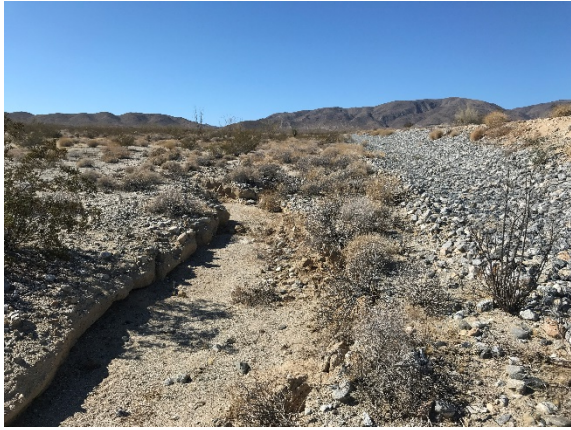
Photograph 5 – Water has cut a channel near the toe of the gabion mattress (Site 5).
