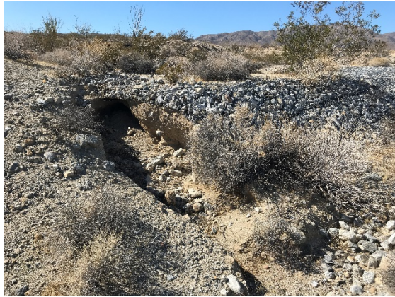
Photograph 1 – Hole below gabion berm undermining structure (Site 1)
