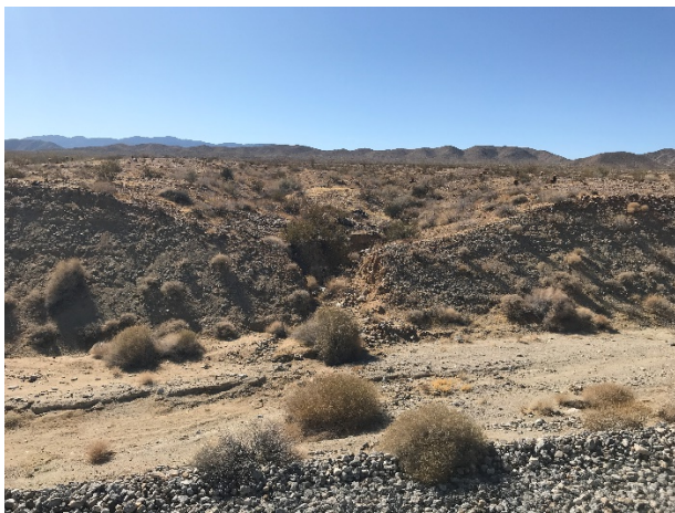
Photograph 3 – Natural gully has eroded earthen berm (Site 3).
