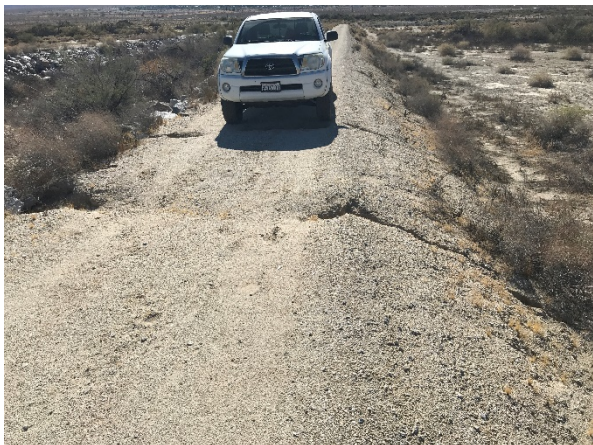
Photograph 13 – Cracks or gully erosion in berm that extend through berm (Site 14).
