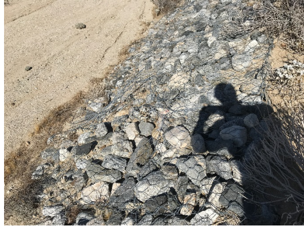
Photograph 6 – Caged gabion material has ripped (Site 6).
