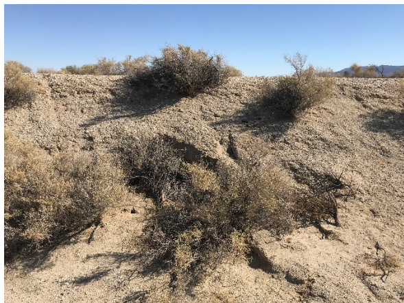
Photograph 11 – Hole in earthen berm (Site 11).
