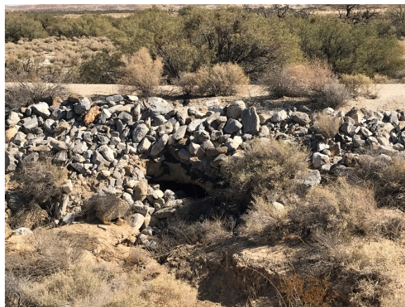
Photograph 10 – Hole at the base of the berm that extends perpendicular through the entirety of the berm (Site 10).
