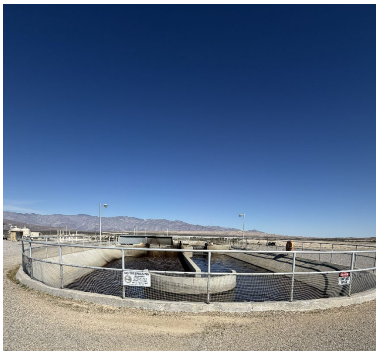
Figure 12. The 250,000-gallon oxidation ditch with brush rotor surface aerators.
