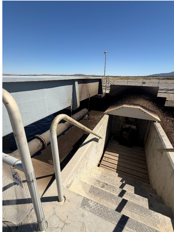
Figure 13. The motor for the brush rotor surface aerators and oxidation ditch influent pipe are shown.
