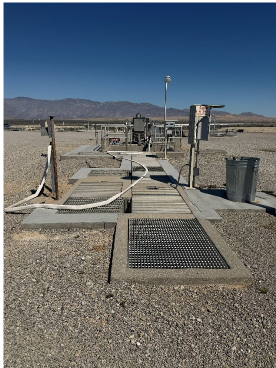
Figure 6. View of headworks which includes a bar screen, comminutor (Muffin Monster), and Parshall flume for influent flow monitoring.
