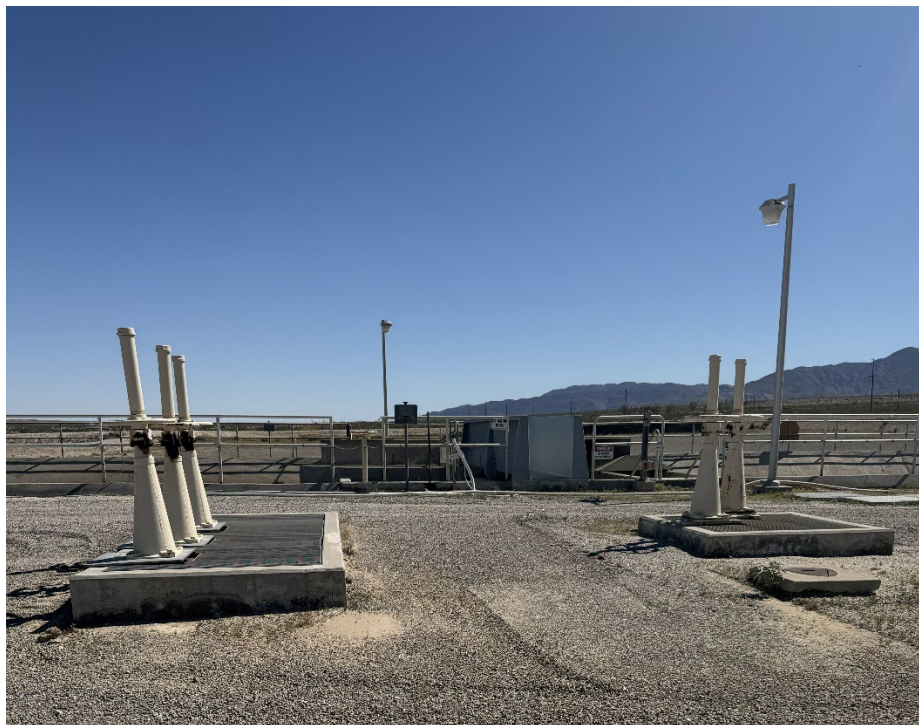
Figure 16. Flow splitter boxes. The splitter box on the right is equipped with valves to control flow from headworks to the oxidation ditch while the splitter box on the left controls flow from the oxidation ditch to the clarifiers.
