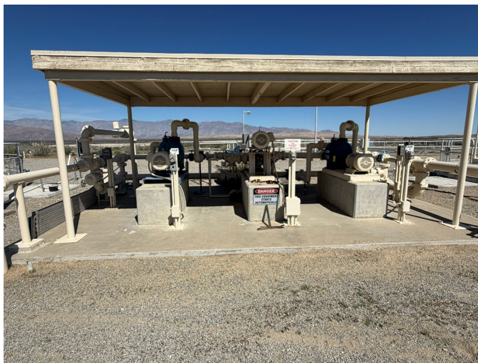
Figure 16. The waste activated sludge (WAS) and return activated sludge (RAS) pumps located between the two clarifiers under a canopy. Sludge from the clarifiers is returned to the oxidation ditch or wasted to the sludge holding tank.
