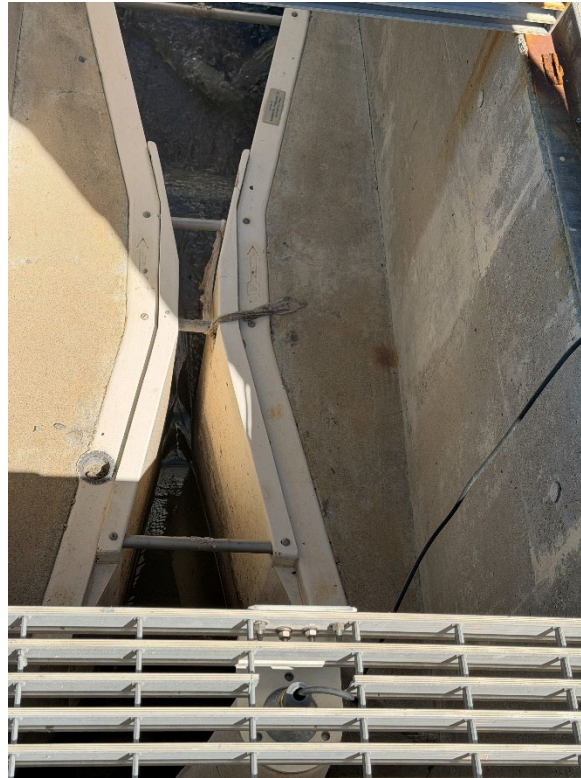
Figure 7. The Parshall flume is used for influent flow measurement. Influent samples are collected downstream of the Parshall flume.
