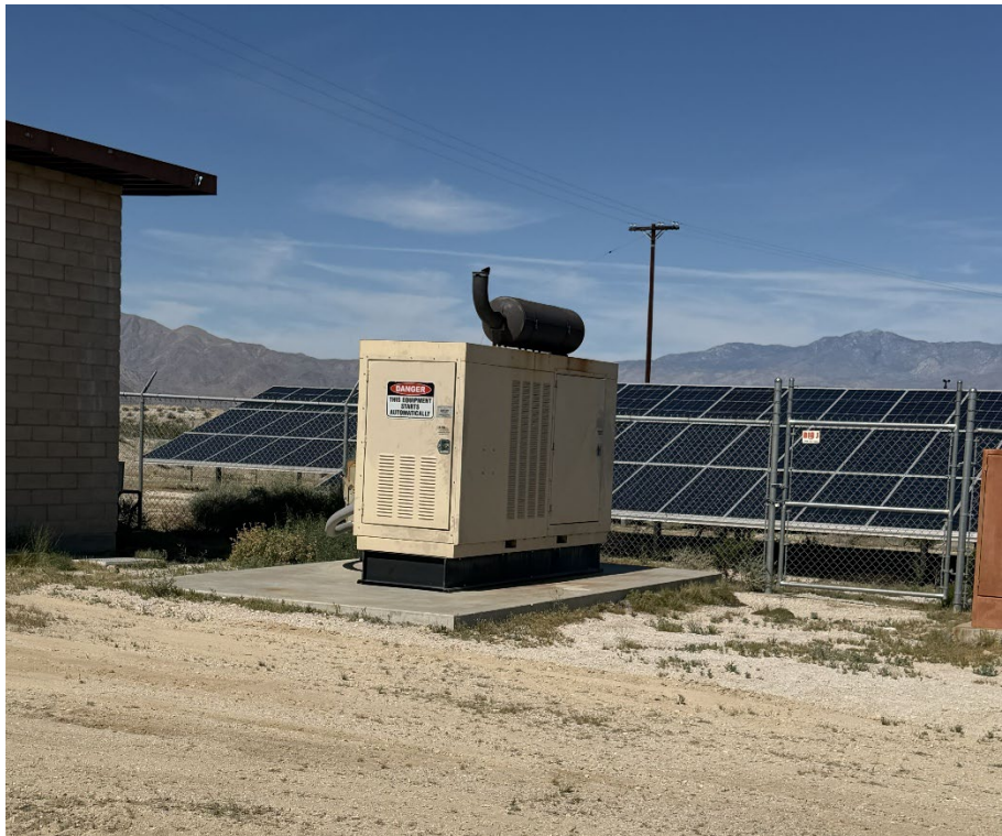
Figure 5. An emergency generator that supplies emergency power to the plant is shown. Solar panels, behind the generator, that provide power to the plant, are also shown.
