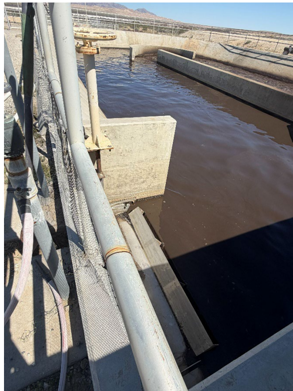
Figure 14. The oxidation ditch effluent weir that can be adjusted by using the hand wheel.
