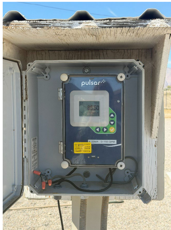
Figure 8. The influent flowmeter display shows current flow measurements. The flowmeter is calibrated once a year.
