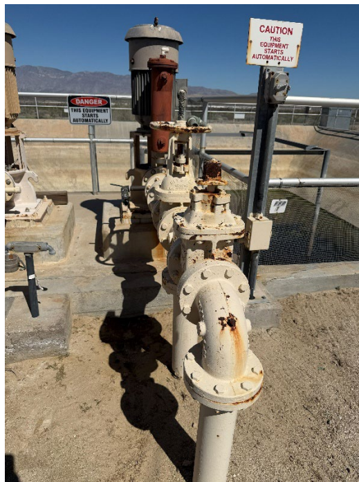
Figure 20. Effluent sampling port is shown at the discharge header with a manual hand lever.
