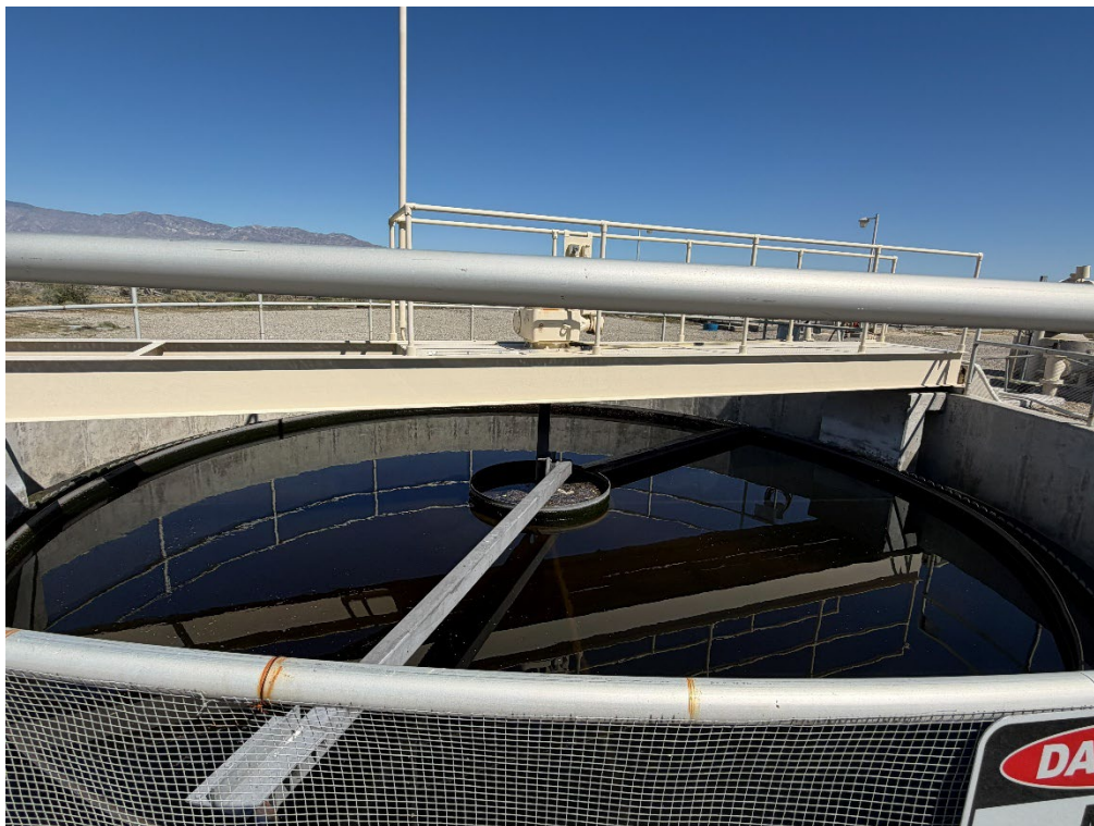
Figure 17. Clarifier 1 in operation during the inspection.
