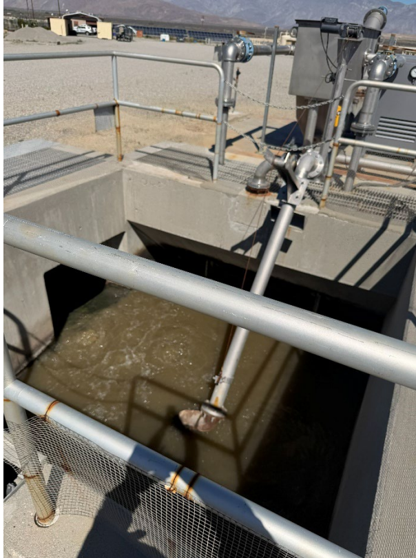
Figure 9. The aerated grit chamber.
