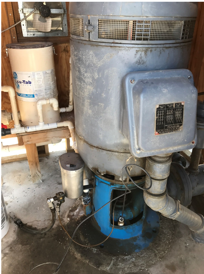
Photograph 1. Well ID1-8 Wellhead and Motor
